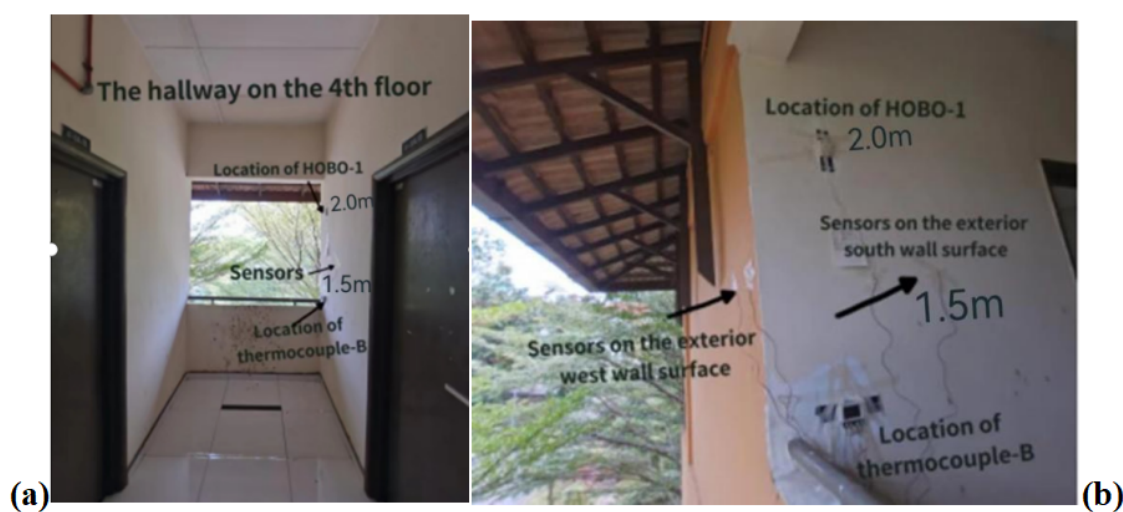
Fig. 4. Images of (a) The installation of the HOBO loggers and thermocouples on the hallway; (b) The installation of thermocouple on the corridor to measure the external surface temperature of the west and south walls.
